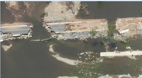
Hillside - Marble Bar Road (severe washout)
