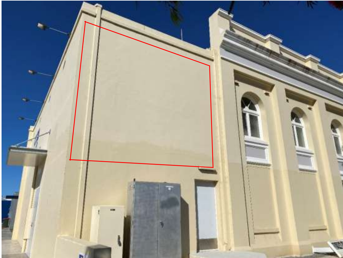
Side view of Gallery (Durlacher St). Mural area is approximately 5 metres wide x 5 metres high.
