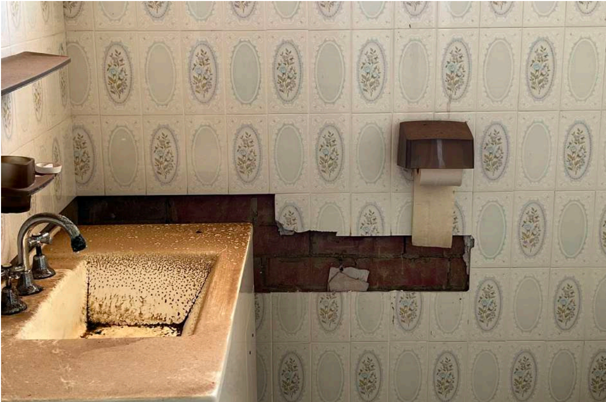
70 Mould and damage to wall tiles in Ensuite
