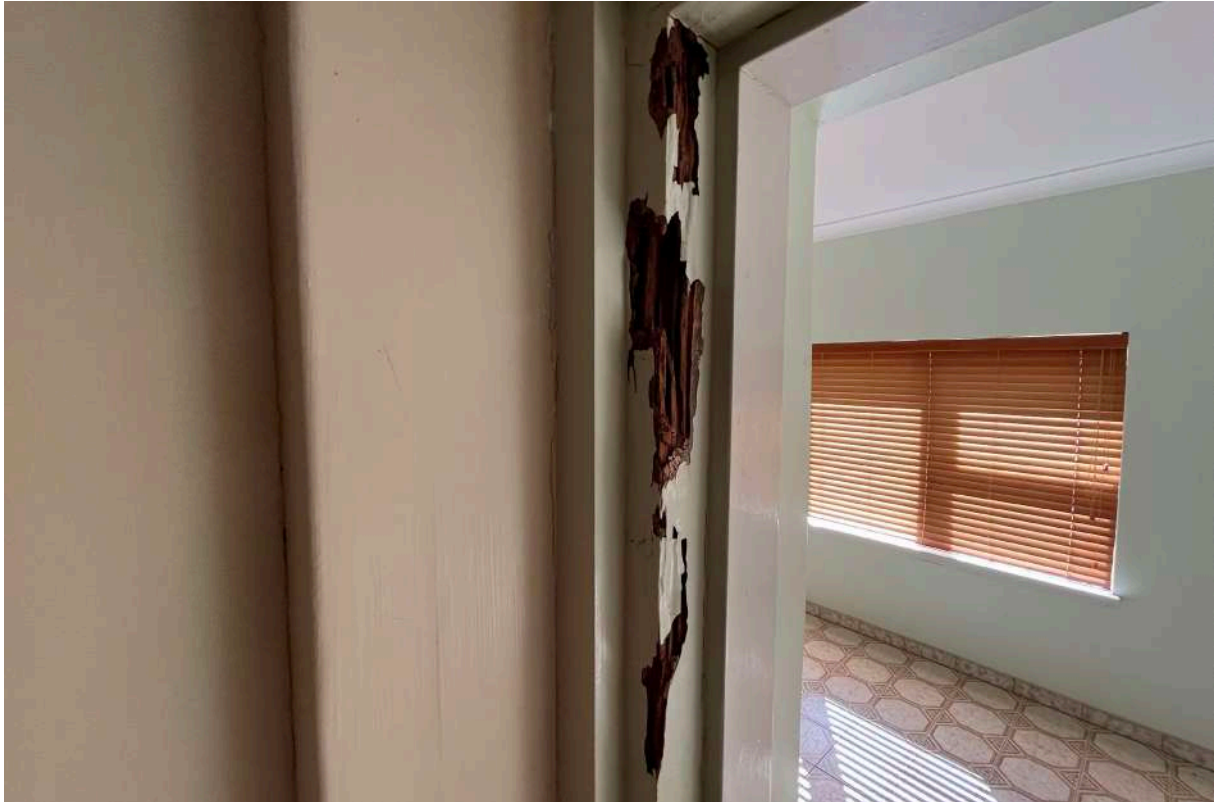
33 Bed 1 door frame termite damage
