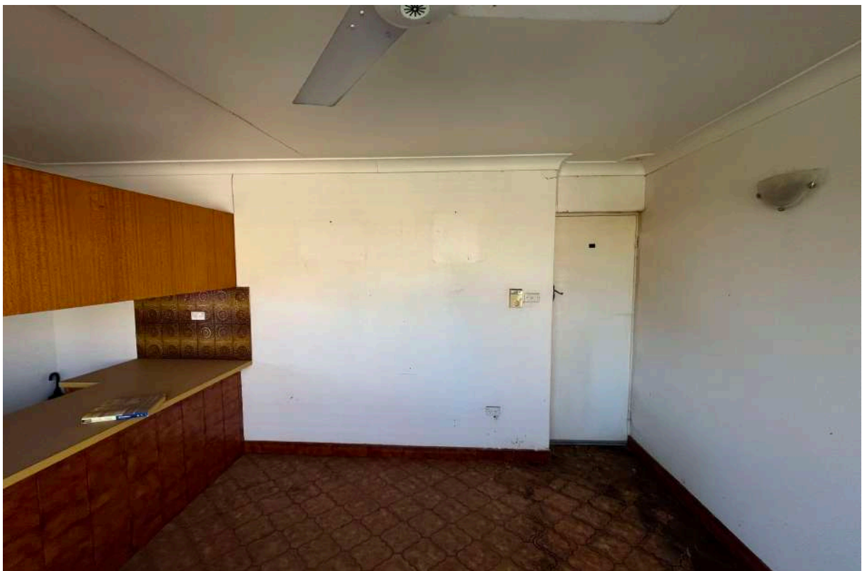
58 Living 5 with floor damage
