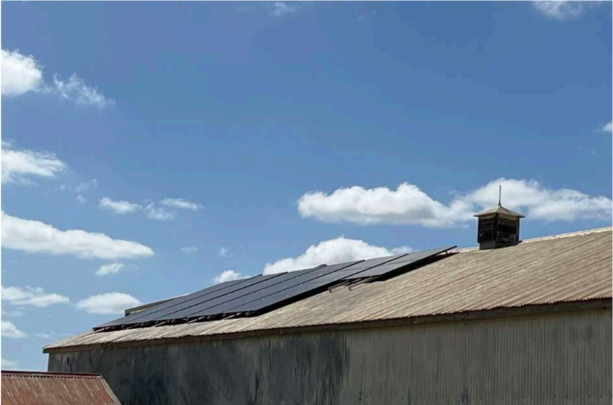
73 Solar panels and cupola to Shed 1
