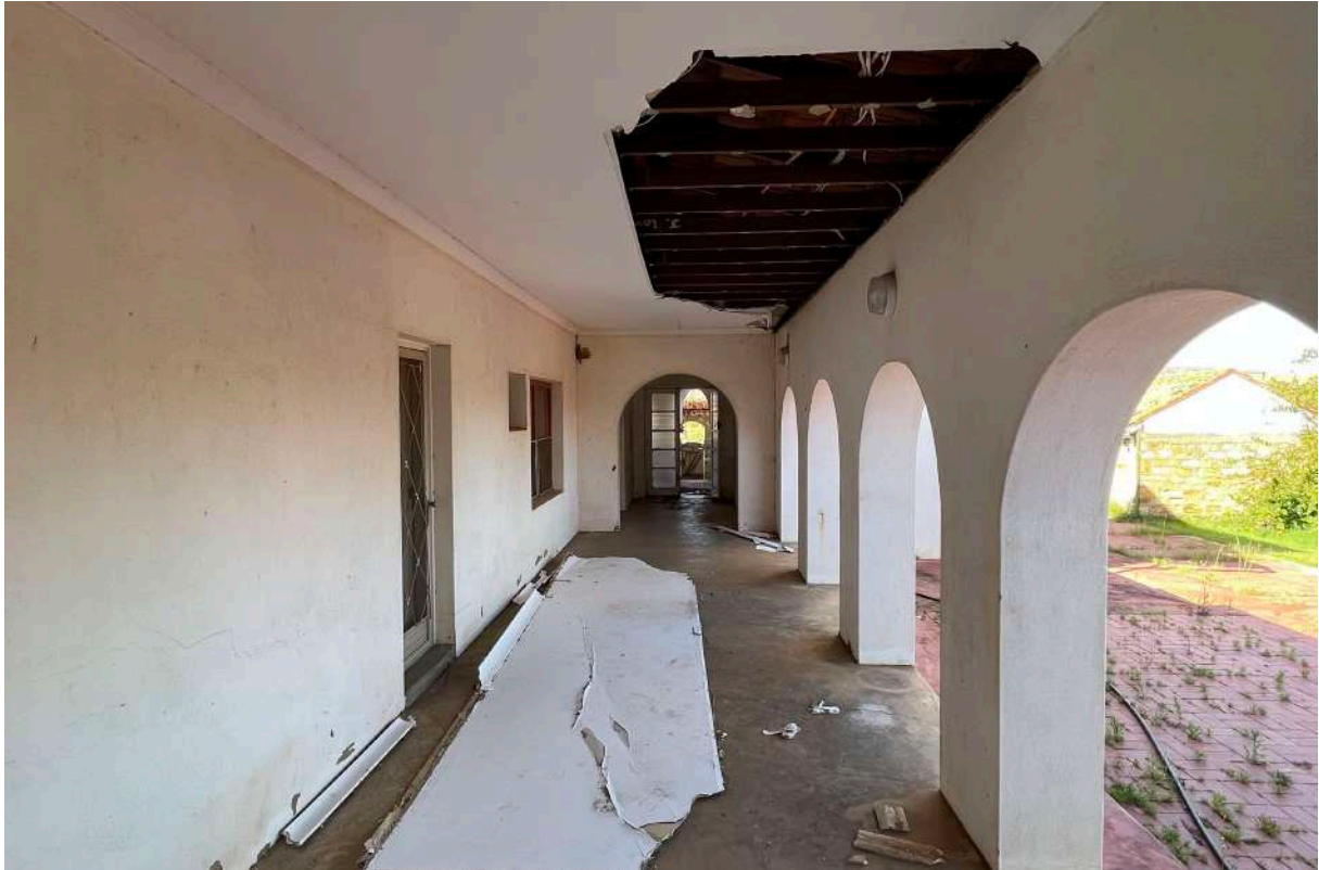
23 Rear verandah with damaged ceiling
