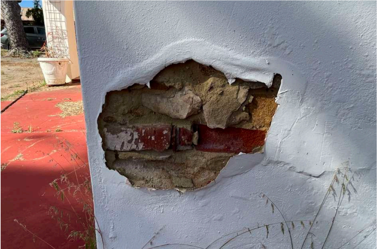
09 Missing render to south west corner
