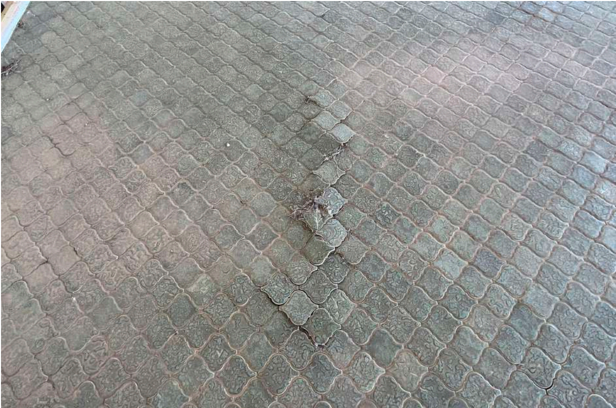
62 Damage to balcony tiles
