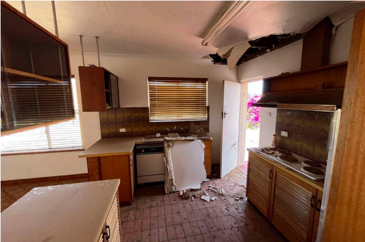
56 Kitchen 2 with damaged ceiling
