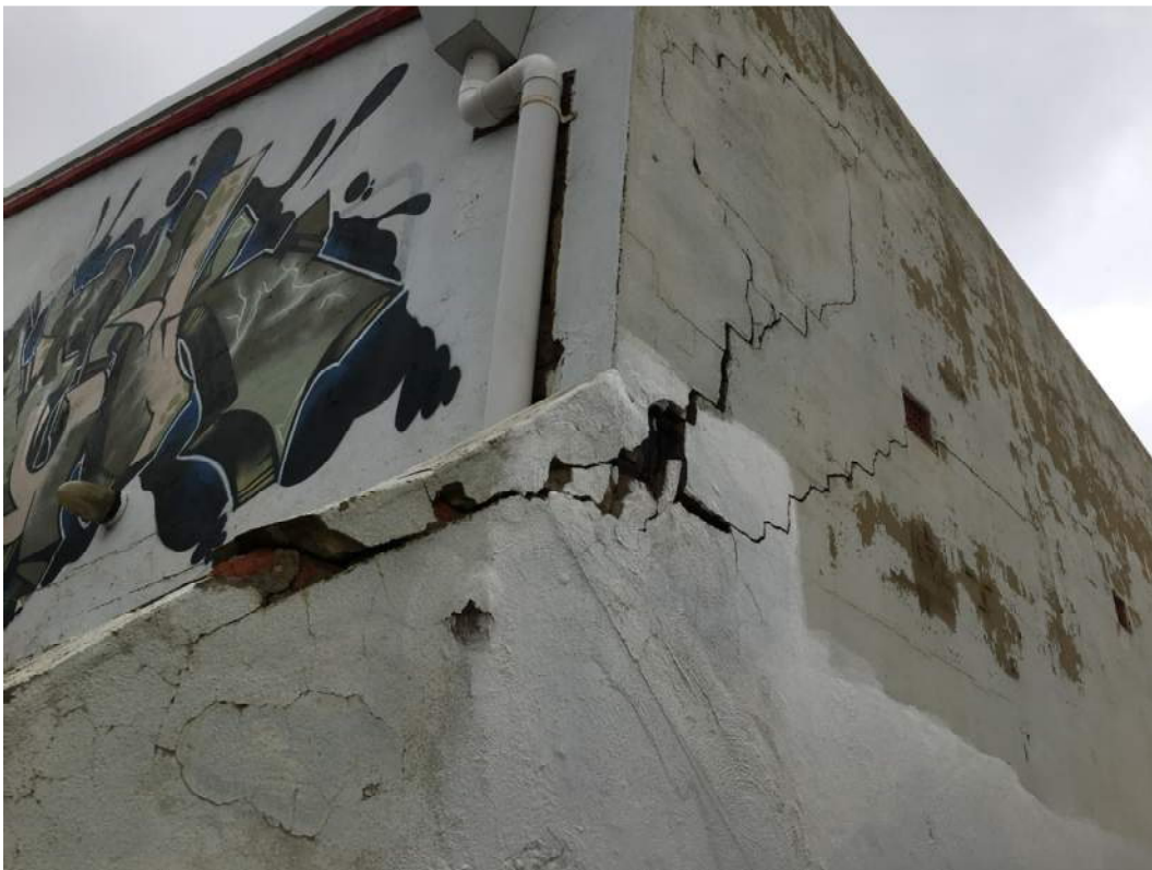
Figure 15: Closeup of cracking of masonry wall on western corner of building
