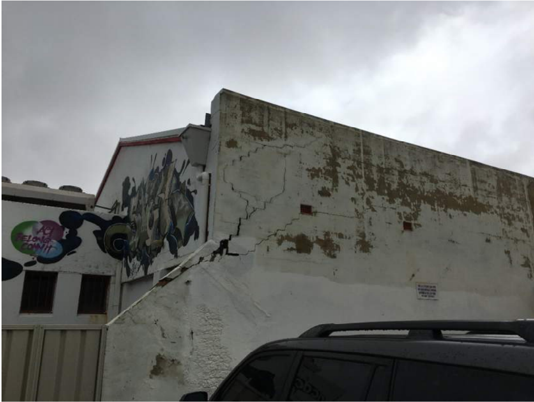
Figure 14: Extent of cracking of masonry wall on western corner of building
