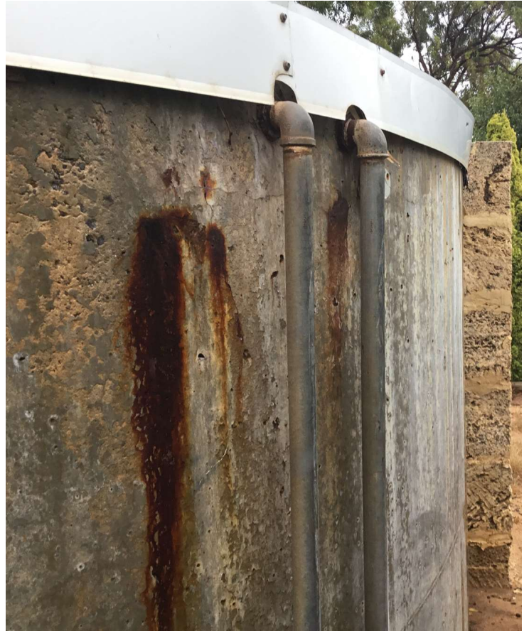
Apex Park Water Tank – severely corroded
