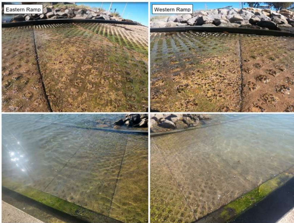
Francis Street Jetty Boat Ramp Waffles requiring renewal
