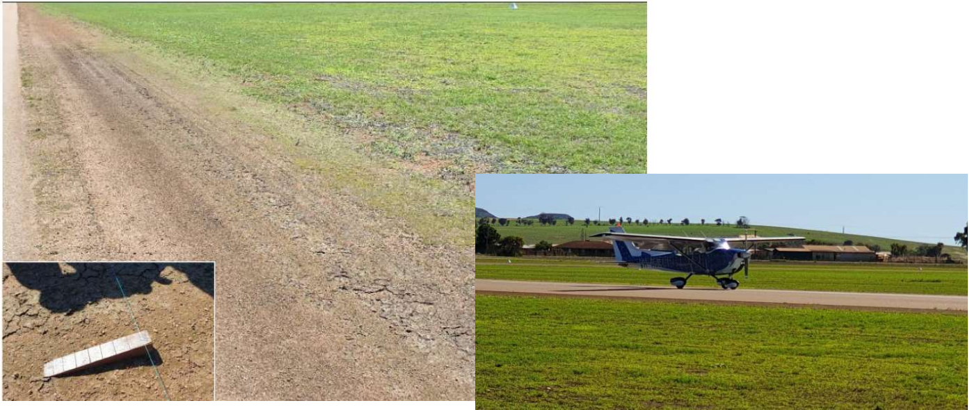
14/32 Runway Shoulder – surface cracking requiring resurfacing works
