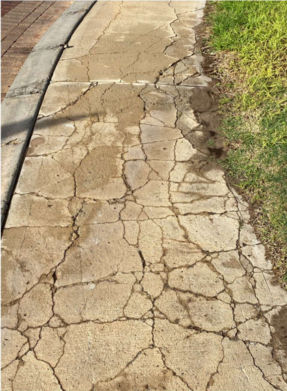
Waterfront Circle, Drummond Cove – path requiring renewal
