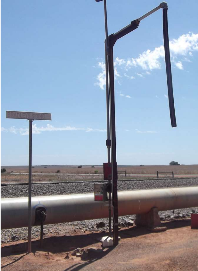
McCartney Rd (Bradleys Siding) Standpipe support renewal required
