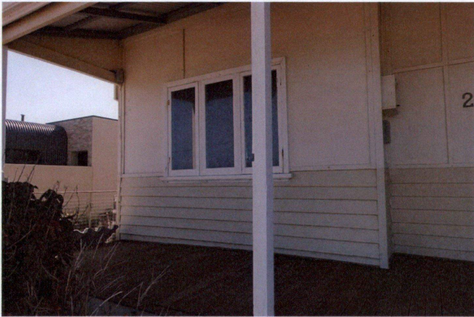
Thrust bay to main bedroom (Room 1) and blocked in front door to the right.
