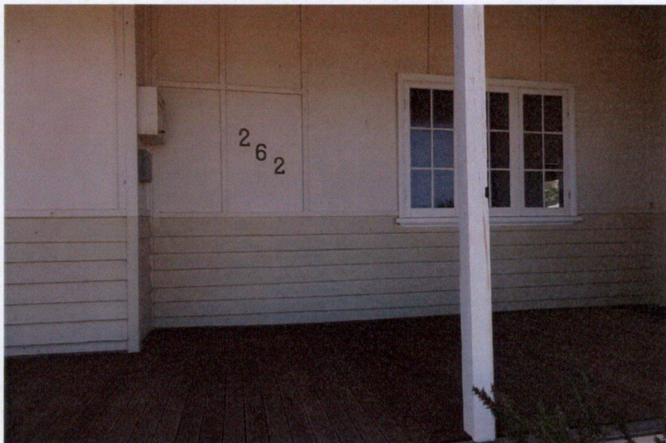
The old front door location and the set of windows that are most likely original.
