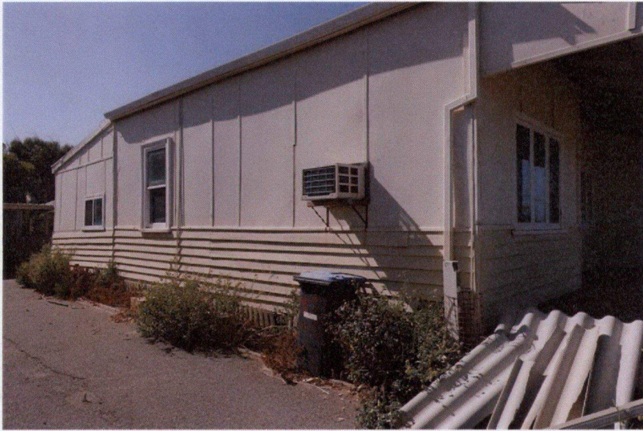
North elevation which is largely original fabric, aside from the window in the skillion.
