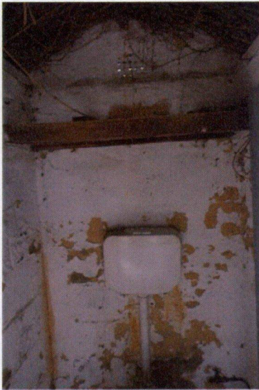
Interior of the water closet and washdown cistern brackets.
