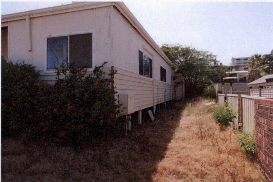
The south elevation, a filled in verandah with aluminium windows. The tree in the distance is a Cape Lilac.
