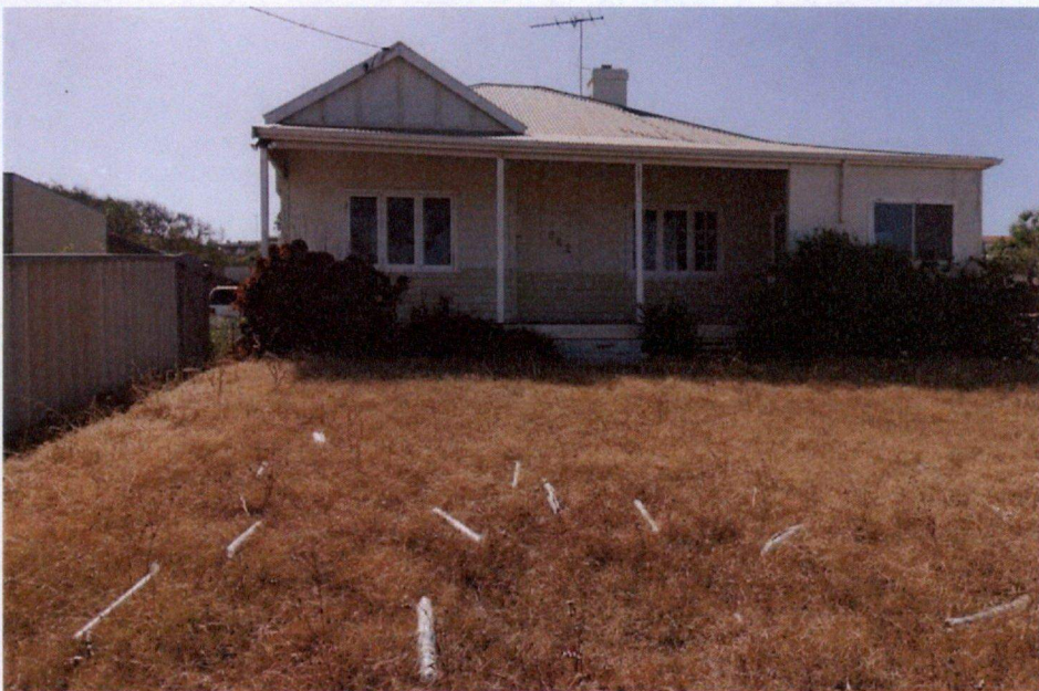
Front of 262 Chapman Road, note the front door was removed and the west and south verandahs filled in. The verandah posts are original and scars on the posts indicate a balustrade.
