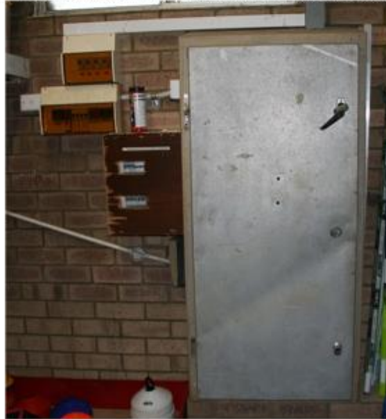
EXISTING CLUBHOUSE SWITCHBOARDS
