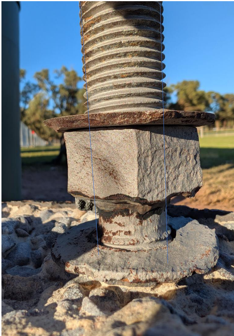
Figure 16: Worst case corrosion of anchor bolts under nut.
