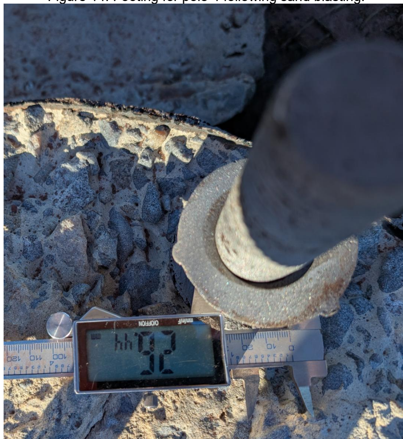
Figure 15: Worst case corrosion of anchor bolts.
