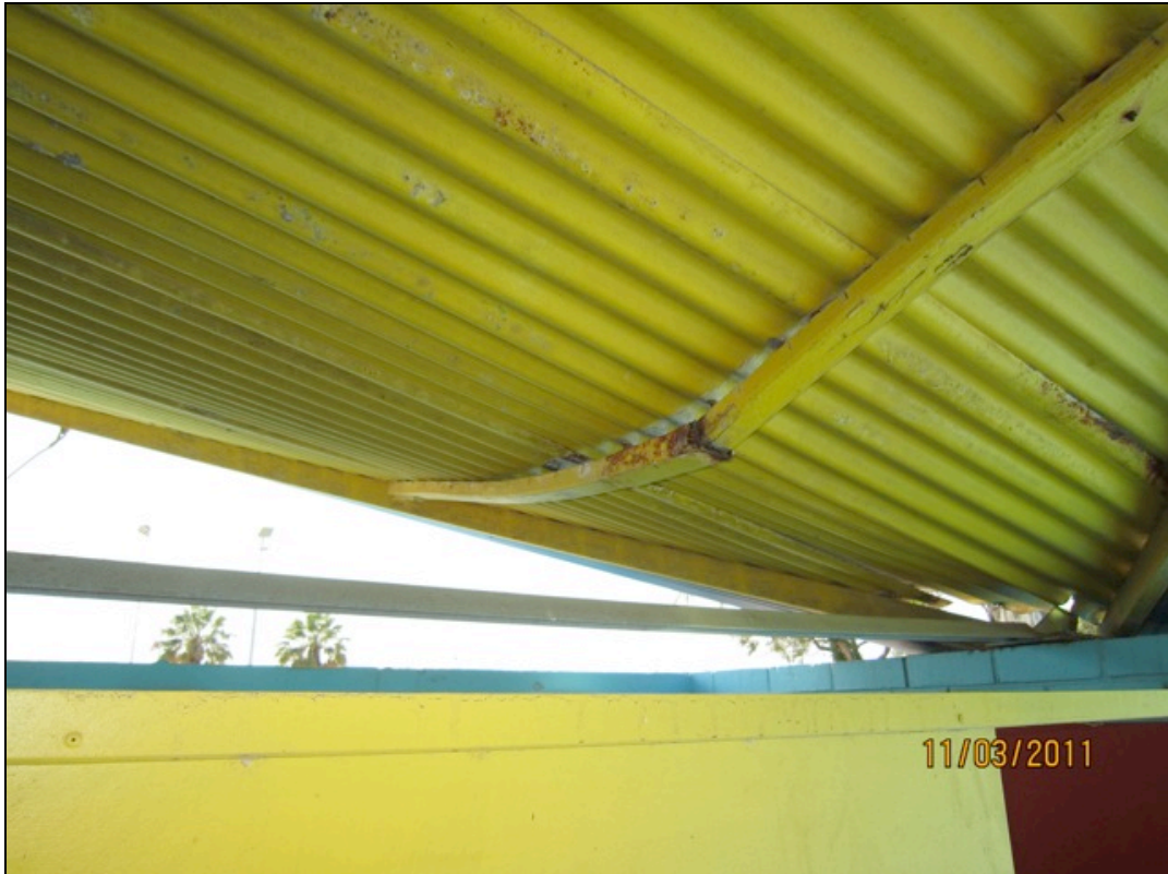
Photograph 3 - Failure to purlin
