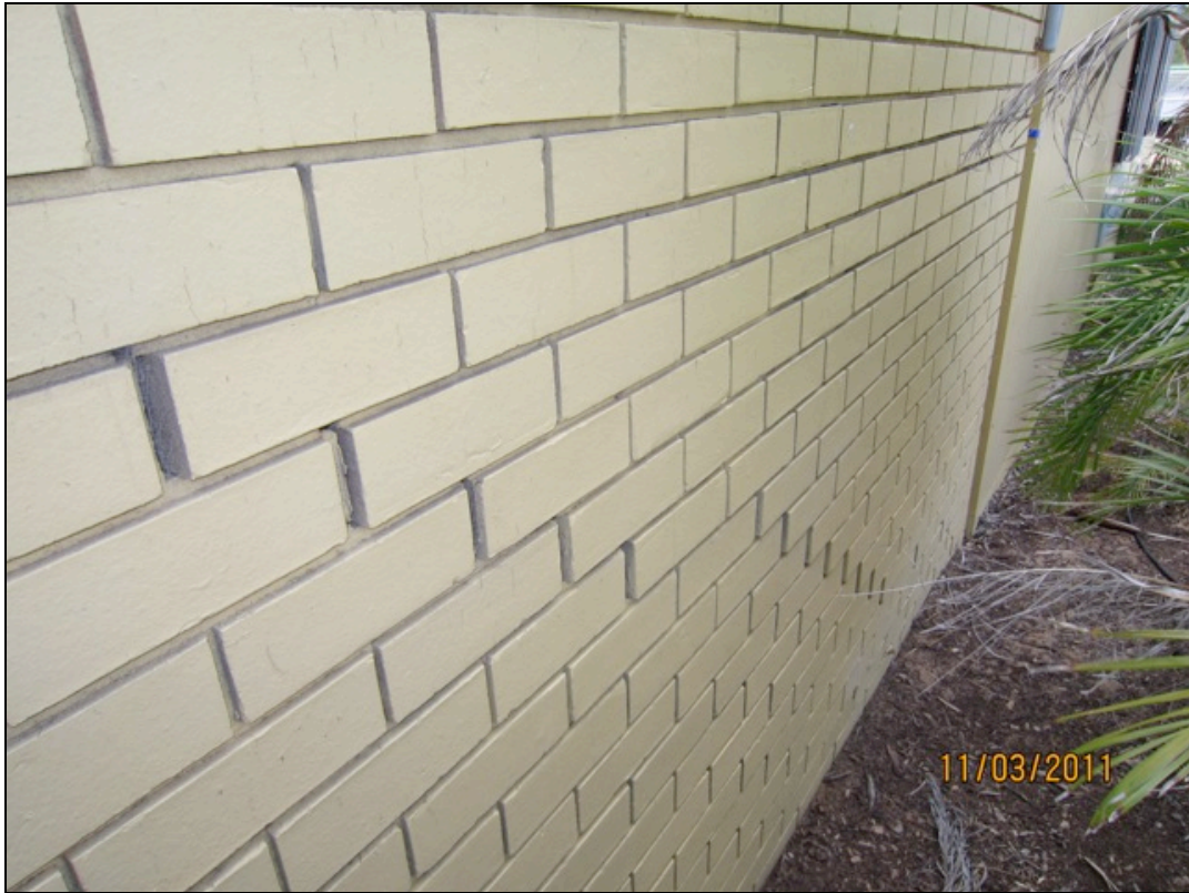
Photograph 5 – Cracking to brickwork
