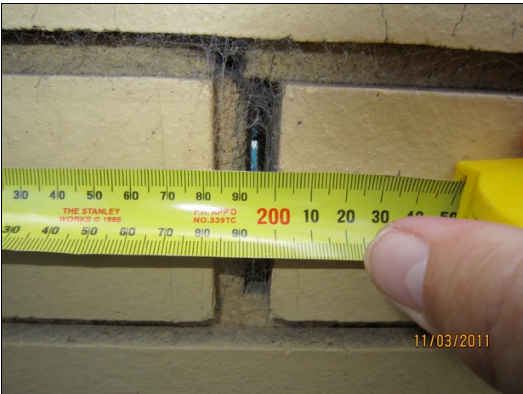
Photograph 4 - Cracking to brickwork
