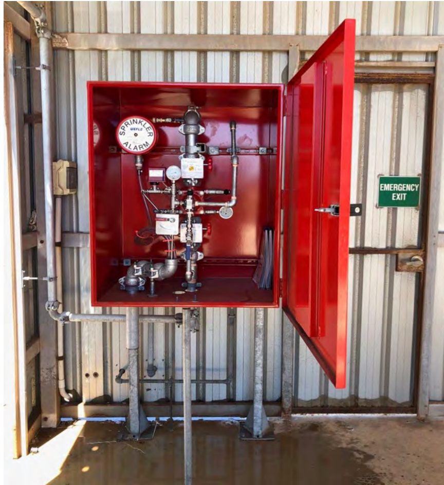
Photo 27 – *Control system for the Store PS1 deluge sprinkler system
