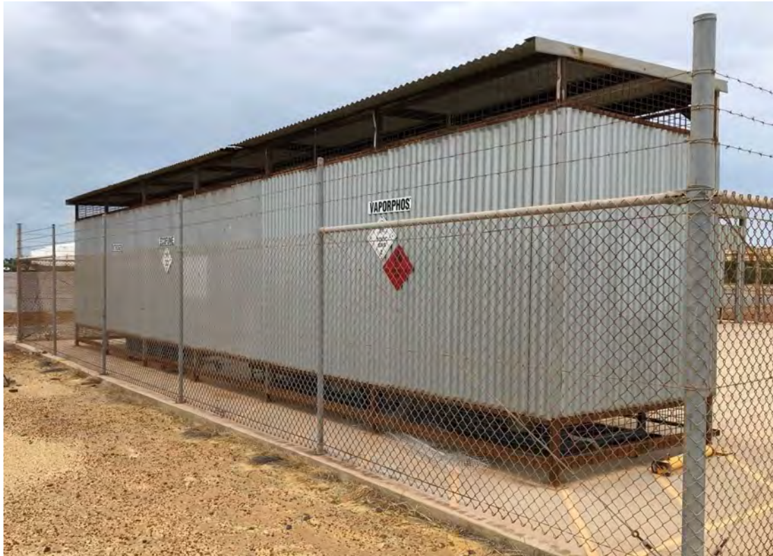
Photo 13 – *Back of Store PS1 showing ventilation, DG placarding and signage
