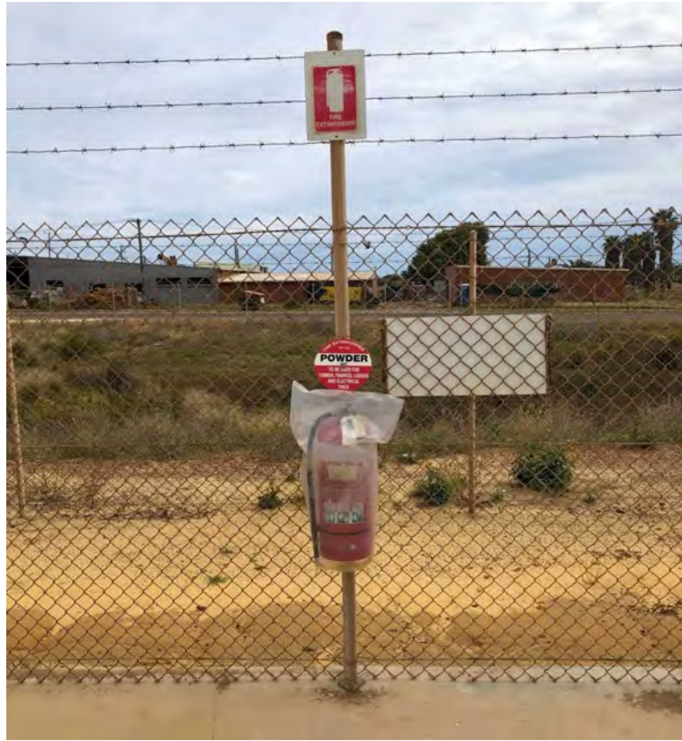
Photo 15 – *FE in the DG compound with signage and plastic cover
