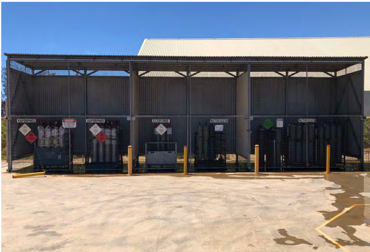
Photo 14 – *Front of Store PS1 showing ventilation, bollards, DG placarding and signage
