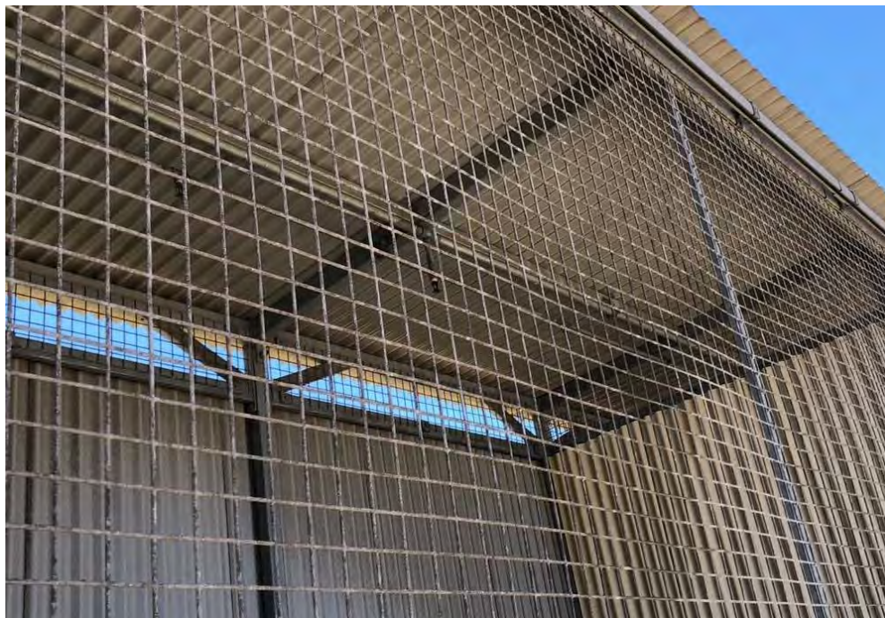
Photo 28 – *Deluge water sprinkler system inside Store PS1
