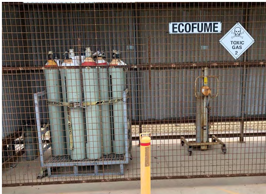
Photo 22 – *Store PS1 showing DG placarding / signage and stillage of EcoFume cylinders
