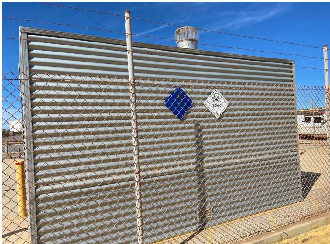
Photo 16 – *Back of Store PS3 showing ventilation and DG placards
