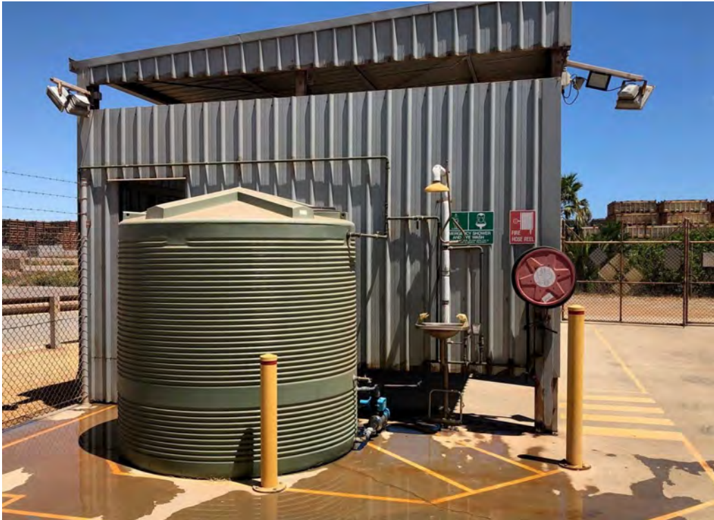
Photo 9 – *Security lighting, water tank, FHR and safety shower / eyewash within the DG compound
