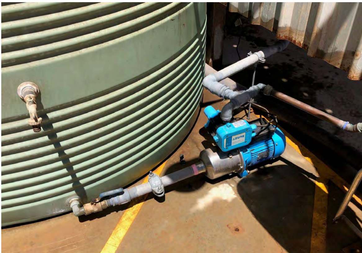
Photo 26 – *Small electric pump associated with the 5,000 L water tank inside the DG compound
