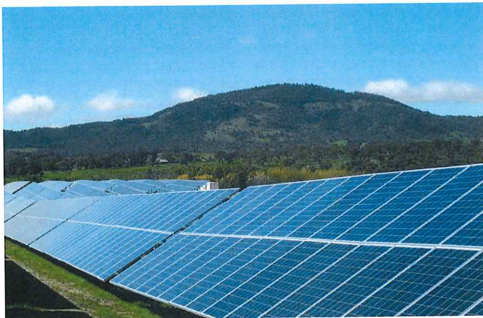
Plate 1: Example of Fixed Tilt solar PV farm
