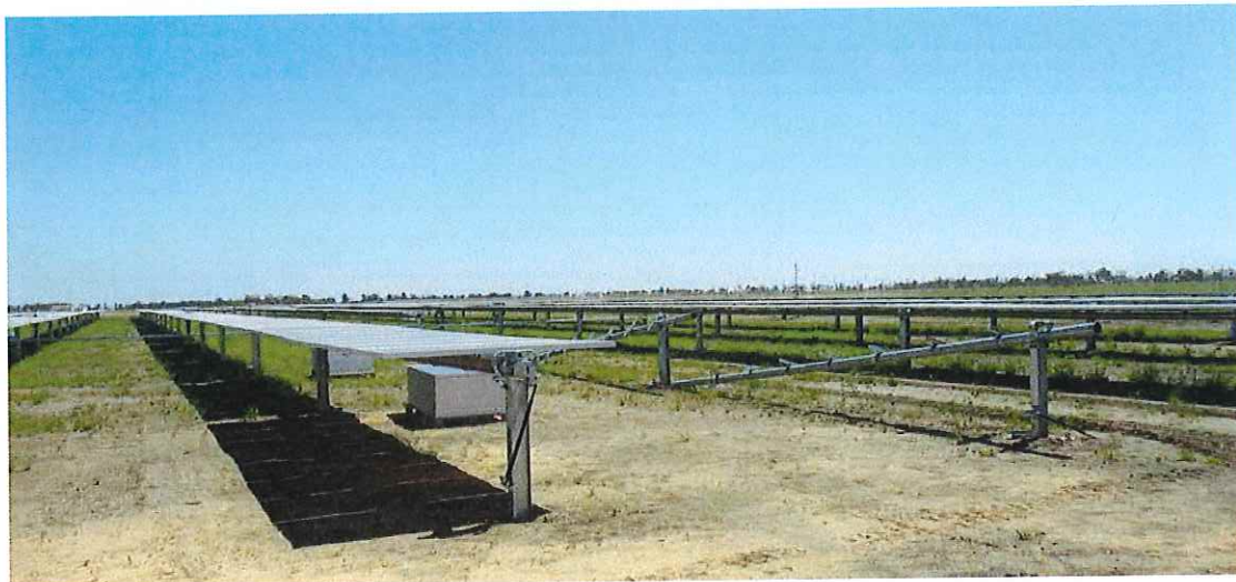
Plate 2: Example of Tracking solar PV farm
