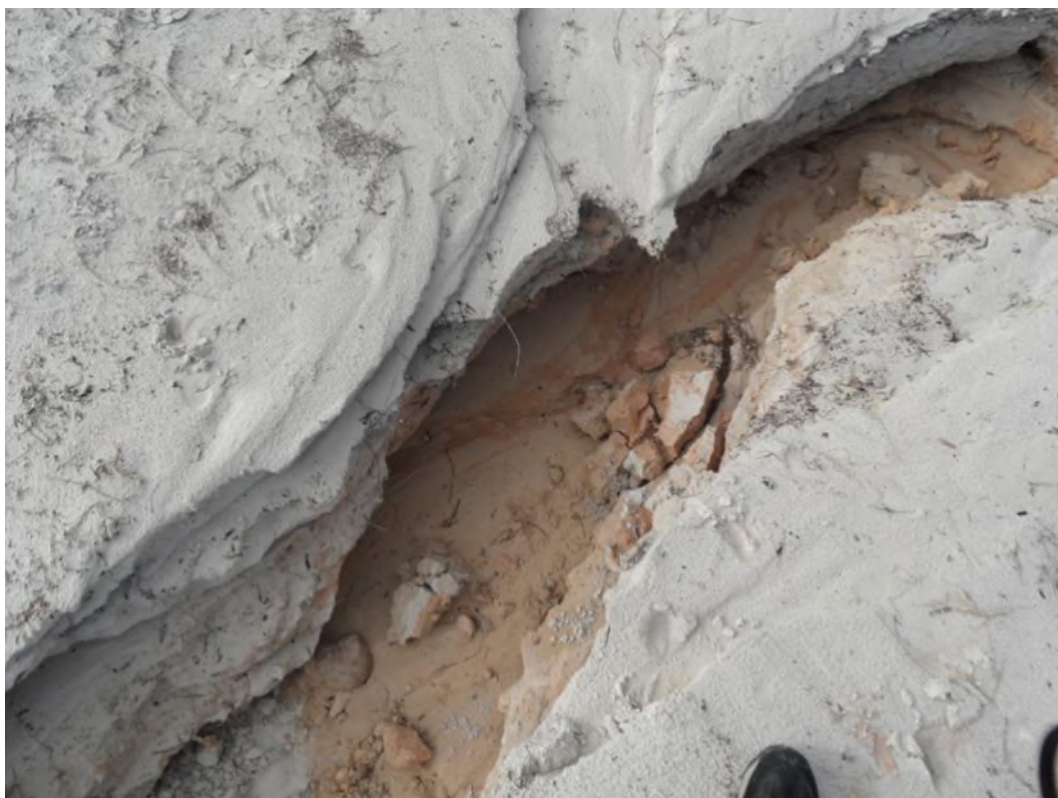
Figure 2.4: Stormwater erosion scarp indicating the vertical variation in sand type at the southern end of the Beresford Foreshore- 30 June 2011
