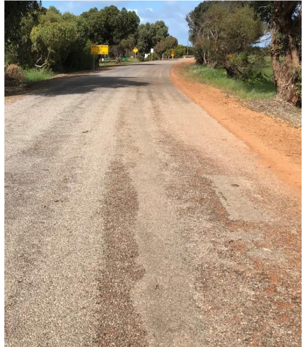
Urban Road Renewal - McCartney Road, Greenough (poor condition)
