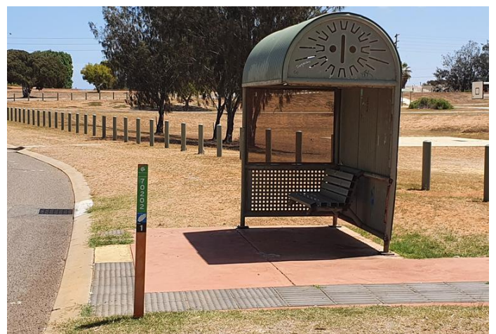
Diosma Bus Shelter renewal due to aged condition
