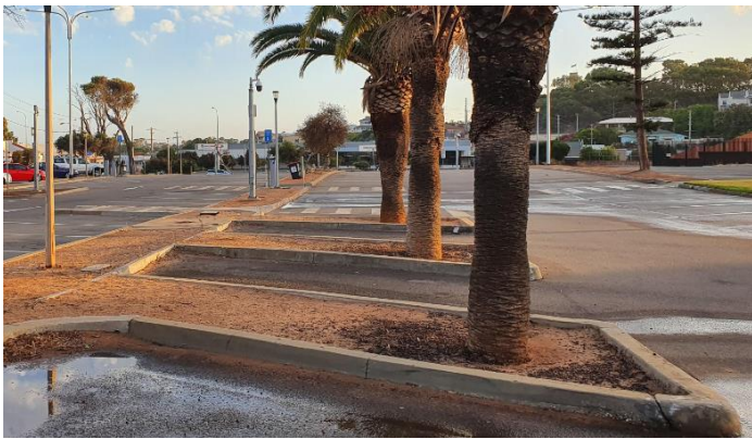
Car park renewal – Sanford Street Carpark Number 5 (islands are bare dirt with mounds creating trip hazards - require landscaping and beautification)
