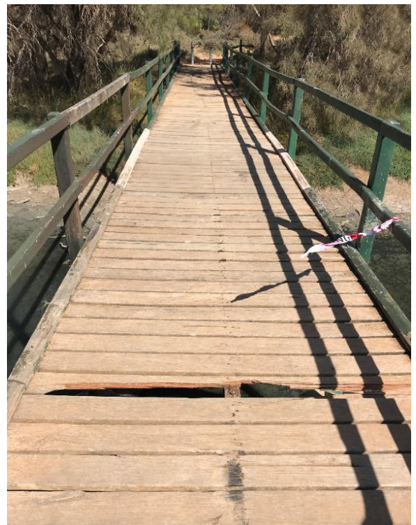
Bridge Renewal - Devlin Pool Pedestrian Bridge (timber deck and railings in poor condition)
