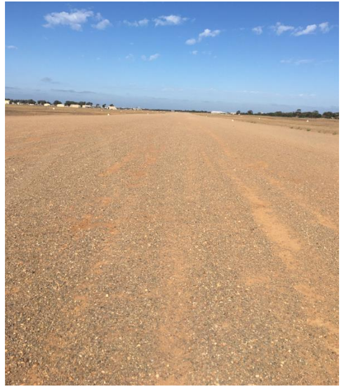
Runway 08/26 – renewal works of gravel runway to grade and reshape the east-west runway. CASA safety requirement.
