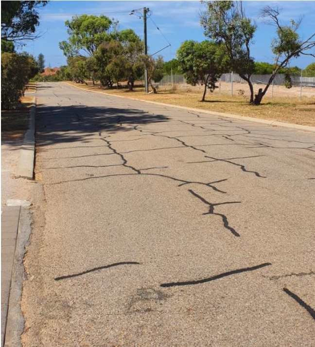
Urban Road Renewal - Baler Road, Sunset Beach (block cracking)
