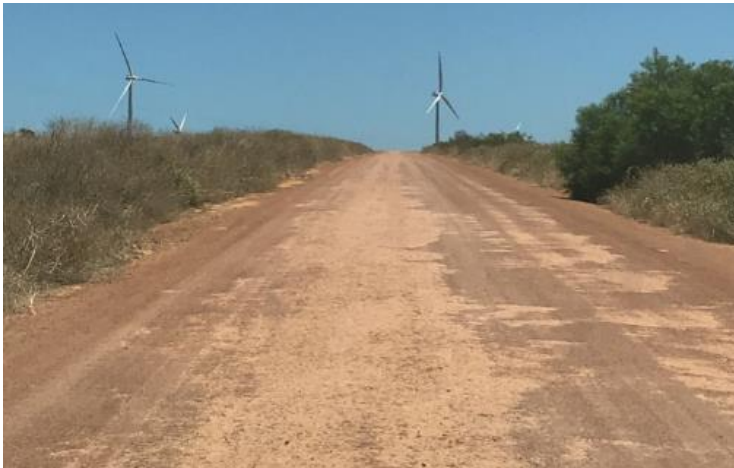
Gravel Re sheeting required William Road
