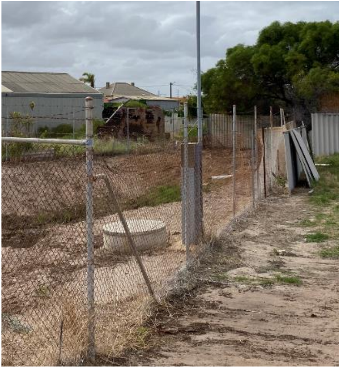
Example of Sump Fence that requires renewal
