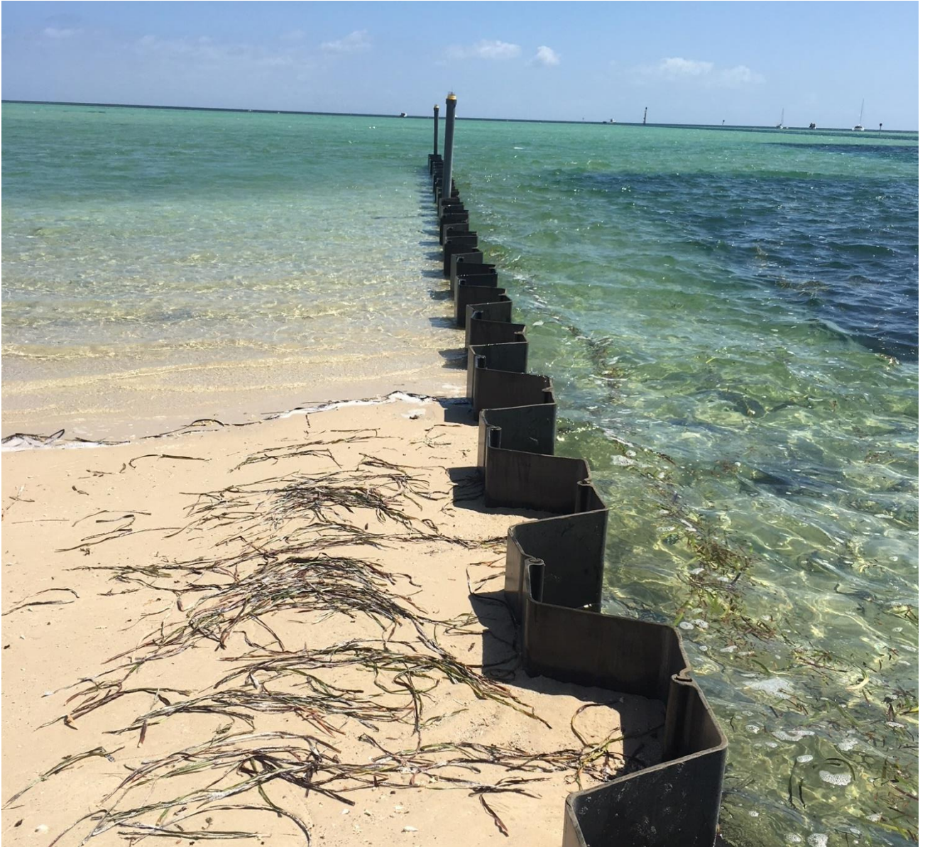
Figure 3.6 Denham Foreshore Composite Sheet Pile Groyne Site Photograph (Supplied by Shire of Shark Bay, 2017)
