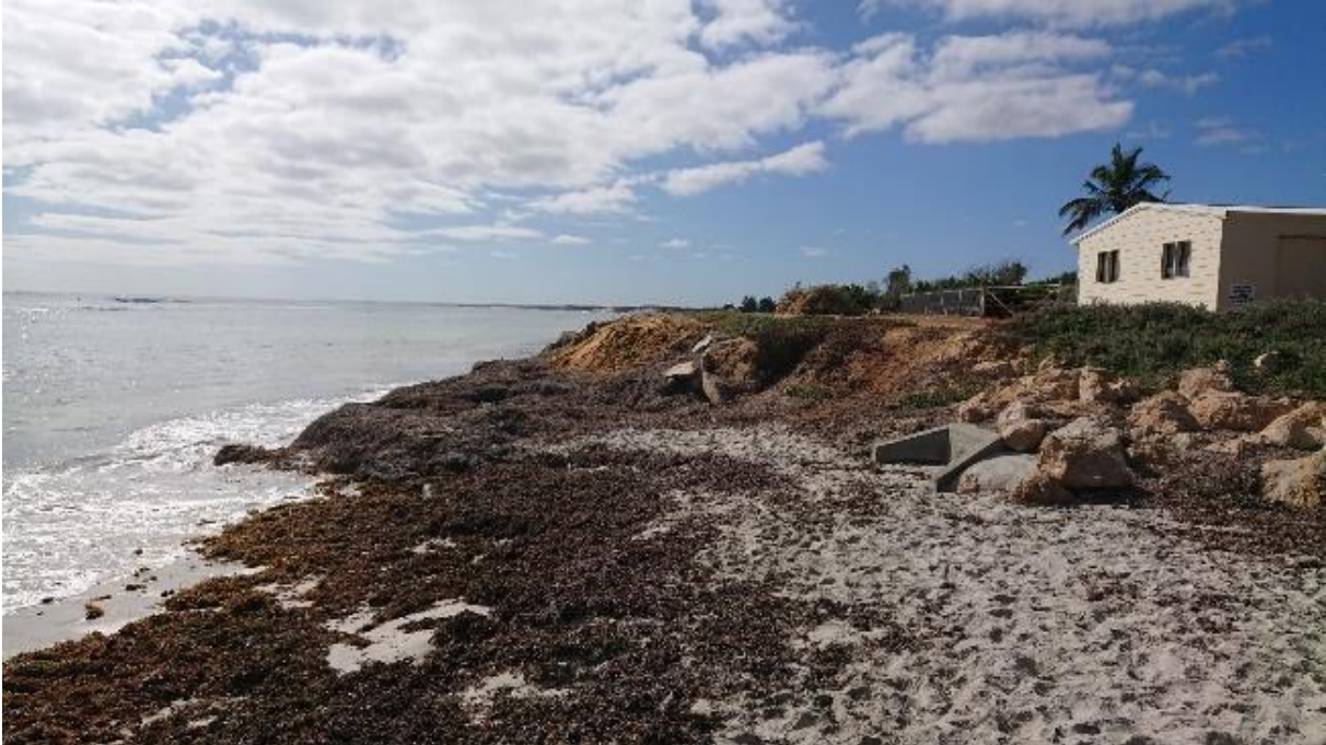
Figure 2.8 Ad Hoc Protection of Freehold Development (far field) and Drainage Infrastructure (near field)
