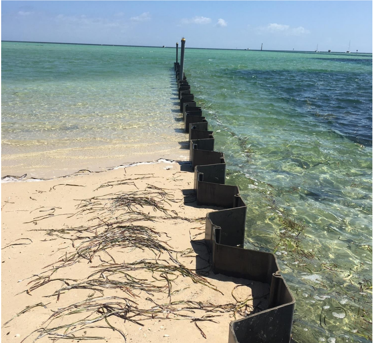
Figure 3.8 Denham Foreshore Composite Sheet Pile Groyne Site Photograph (Supplied by Shire of Shark Bay, 2017)
