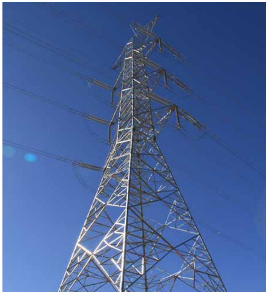
330kV transmission line, Three Springs
