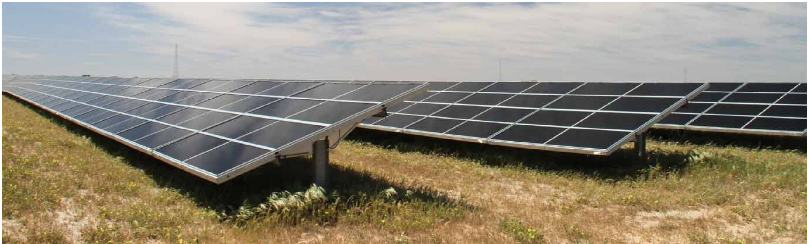
Greenough River Solar Farm, Walkaway
