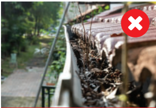
Unmaintained gutter filled with flammable material.
